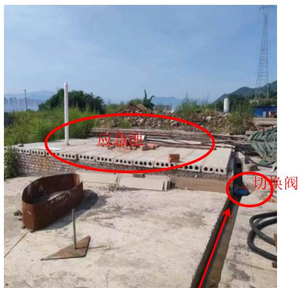
应急处理池及切换阀
